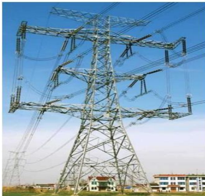
Figure(3-3) Switch Towers
