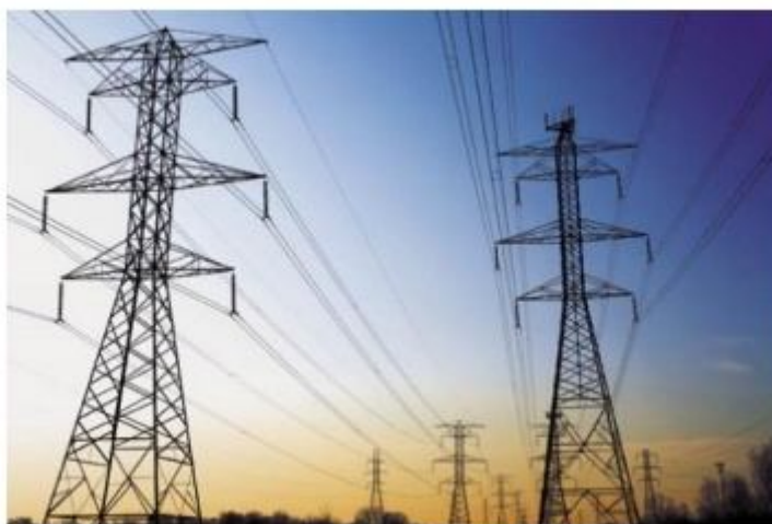
Figure (3-1) Suspension Towers
