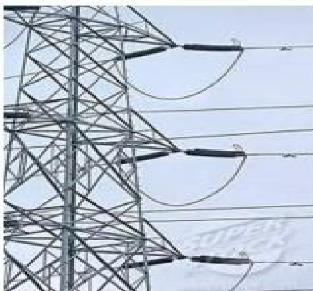
Figure (3-2) Tightening towers
